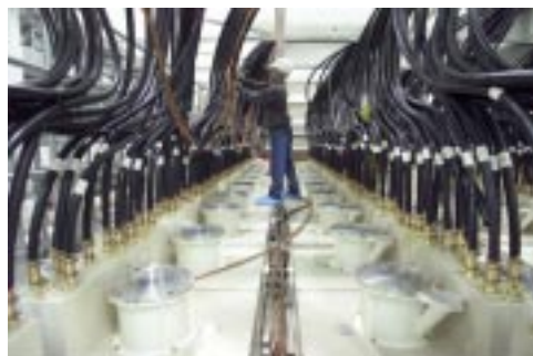
Cables from capacitors to excite laser amplifiers.
