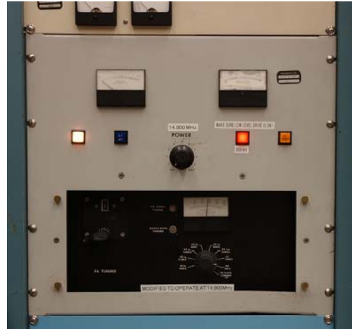
Fig.15 2.5kW generator in operation
